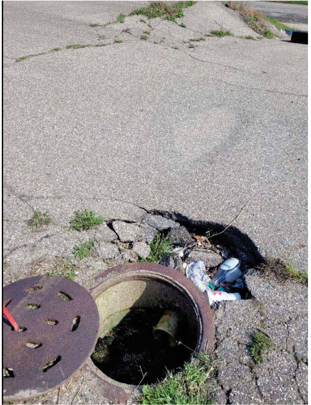
Curb Basin in street with cut black flexi & rough patch in wall where probable bulkhead is.
